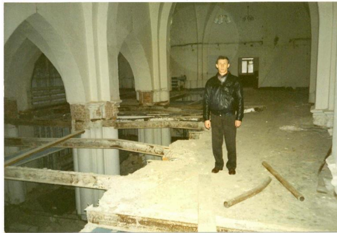
We received the church back on January 1, 1994. Andre Popok, Trustee, oversees the demolition of the archive floors.
