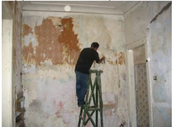
Wallpaper to be removed and walls spackled.
