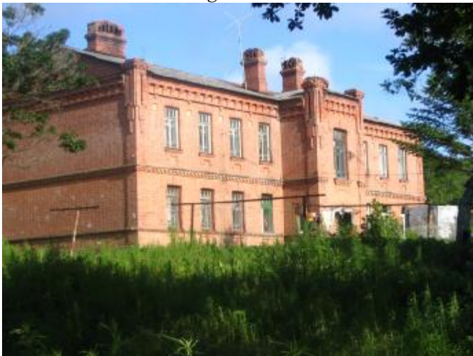
The Retreat house needing work on Russian Island
