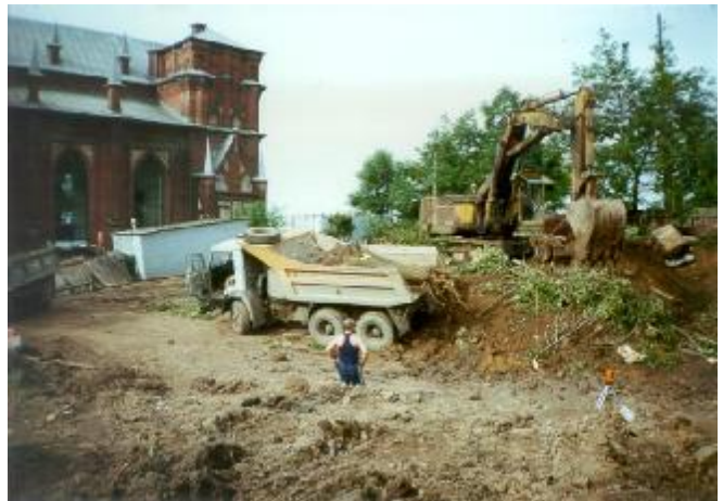
The construction site for the Our Lady of Fatima Rectory and Parish Center.
