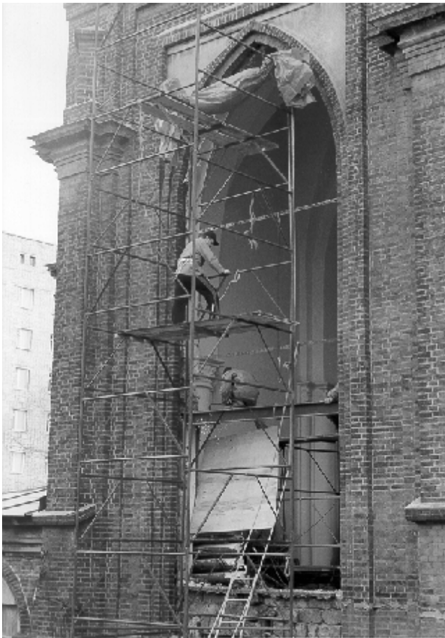
The gaping hole where the new window of the Annunciation will be placed.
